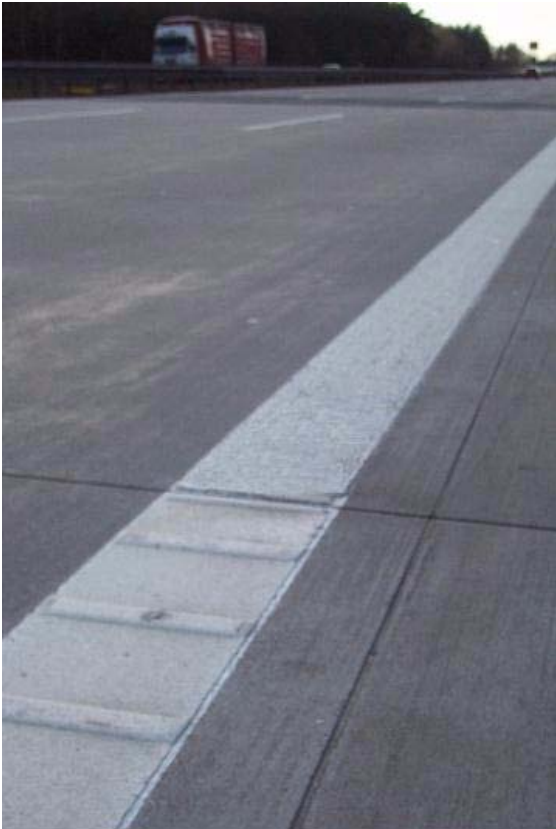
Cross point border marking CP profiled/ CP Agglomerate on freeway A 2 at day, direction Hannover, km 5,0
