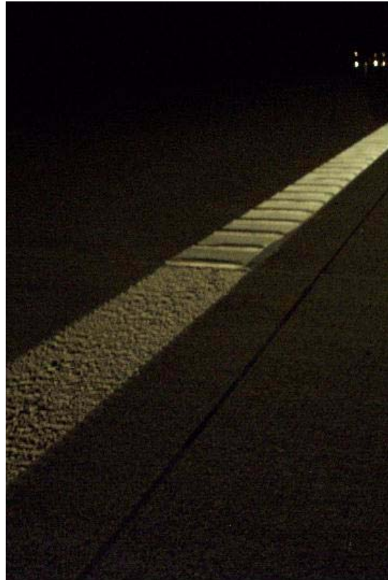
Cross point border marking CP Agglomerate/ CP 90°cross-profiled on freeway A 2 at night, direction Hannover, km 13,5
