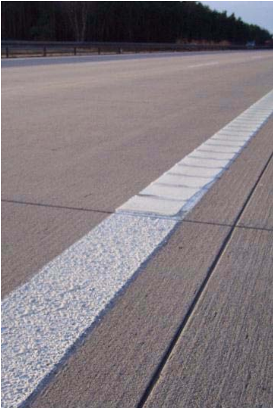
Cross point border marking CP Agglomerate/ CP 90°cross-profiled on freeway A 2 at day, direction Hannover, km 13,5
