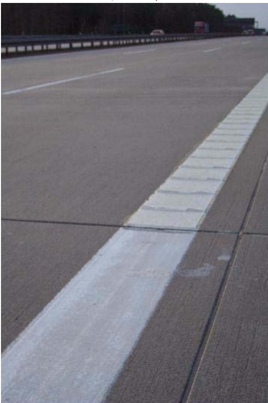
Cross point border marking Paint/ CP 90°cross-profiled on freeway A 2 at day, direction Hannover, km 15,3
